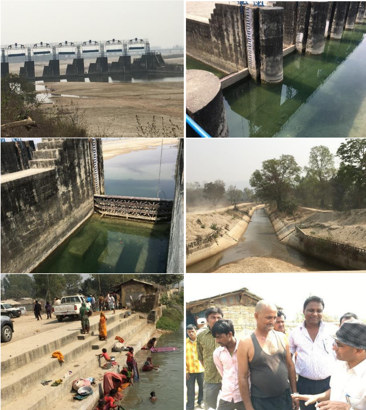
Figure 8 Infrastructure to divert water from the river to the irrigation canals. The water is mainly used for irrigation, domestic, and recreation. Discussion with the communities' leaders and the Head of the Irrigation Division on how water has been used and limitations
