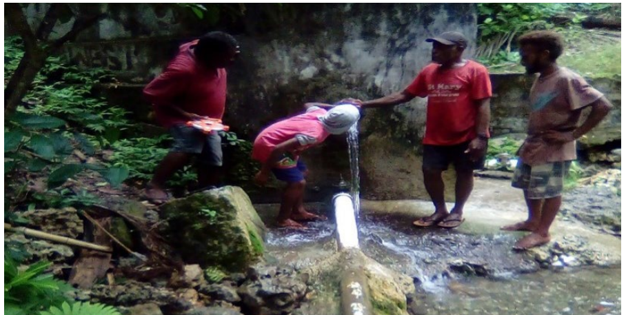
An enclosed storage tank with a pipe that transports water to the village. Water is collected in a spring box and then piped into a storage tank. These types of structures are typical in most of the project communities. Image credit: Water for Women, Solomon Islands
