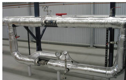
'U' bypass for shutdown/startup/hilly seabed simulations.
