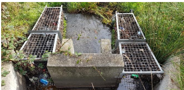
Figure 4: Example of a gross pollutant trap (GTP).
