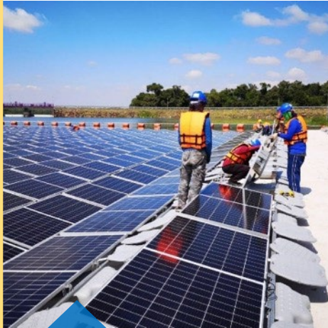
Inverter & Transformer Floating System
