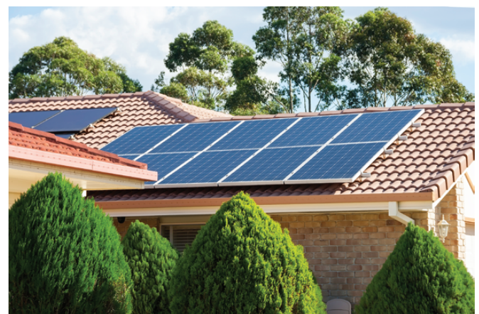
FIGURE 2 Solar PV system (approximately 2.8 kilowatt peak) on a residential rooftop. (chinasong/iStock)
