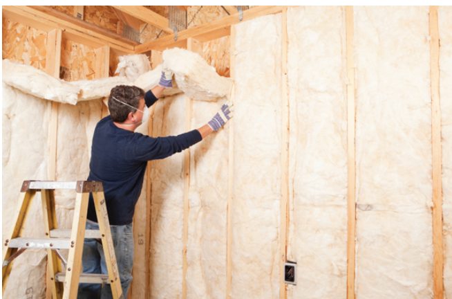
FIGURE 4 Porous sound-absorbing material should be added to wall cavities and roof spaces to deaden sound reverberation. (BanksPhotos/iStock)
