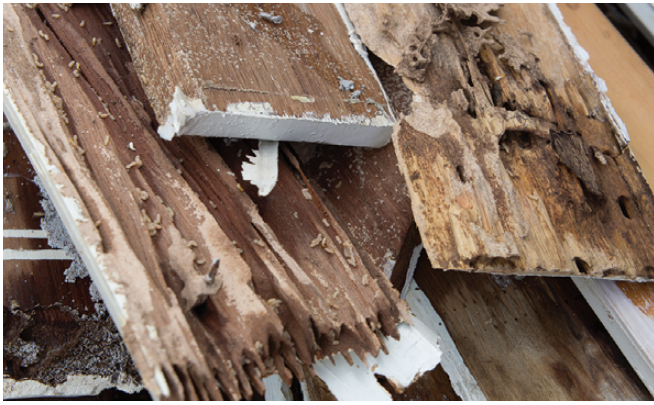
FIGURE 6 Termite damage in wood. (iStock.com/Pixygirlly)
