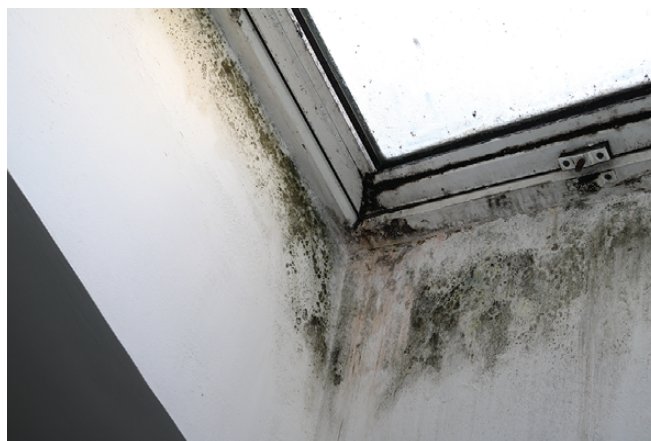
FIGURE 5 Mould growth from persistent indoor condensation near a window. (Ivelin/Shutterstock.com)
