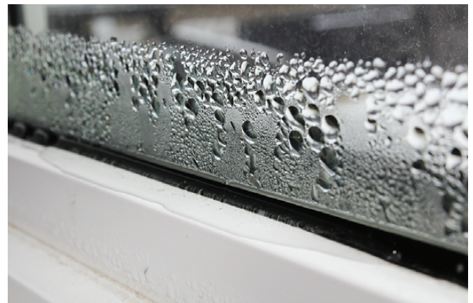
FIGURE 1 Condensation forming on the inside of a window and pooling on the frame. (Amelia Martin/Shutterstock)
