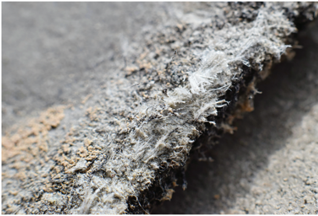
FIGURE 4 Asbestos fibres visible on severely weathered roofing. (Tunatura/Shutterstock)
