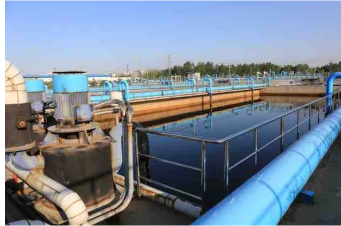
Florida water treatment plant (Feb 2021)
